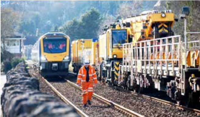
Day 6: Following re-railing of the stricken diesel unit, Network Rail's self-propelled Kirow crane has re-assembled the crane train. Northern's rescue 'tractor' unit is arriving on site behind a Person-in-charge, at walking pace, through the Engineer's 'possession'. (In such circumstances, NR's Engineer is in charge of the railway from Kents Bank to Holme Island.)
